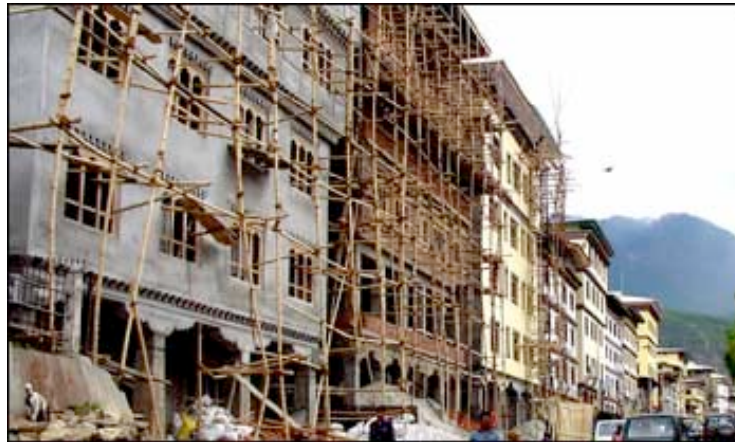
Safety signs are not displayed at work sites
